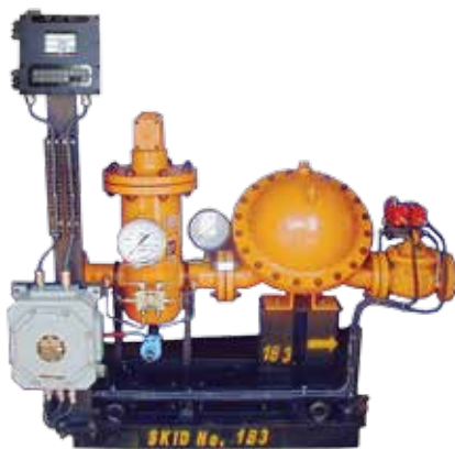
MSA meter skid with Toptech SMP controller
